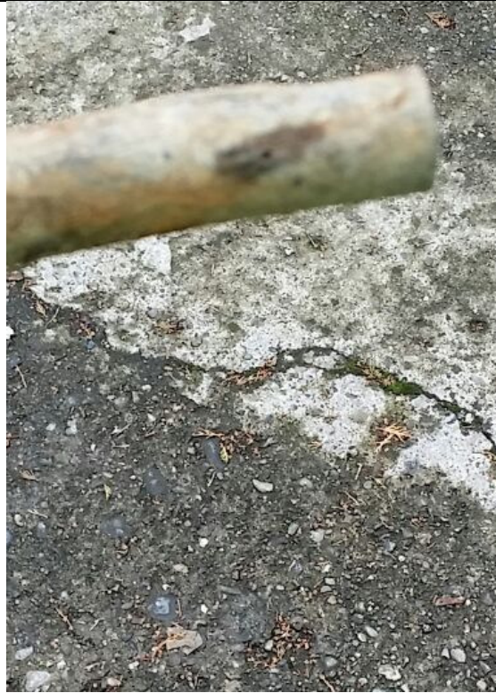
Fine Spray 1.4m 3 Leak – Rubble Infill
