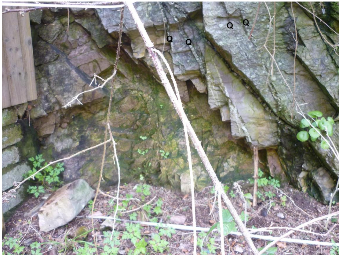
Fig 13.18. Detail of part of Fig. 13.17 showing intense jointing in the Gyleen Formation Glen Road Quarry (middle), Monkstown.
