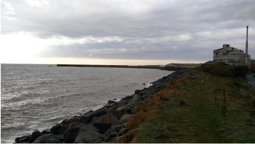
Figure 2.9: Irish Sea and existing revetment adjoining the Old Wallboard site (viewed from the existing revetment to the west of the site)
